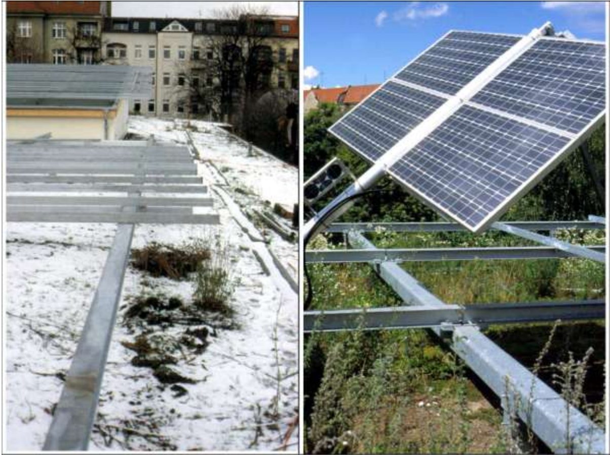
Figure 1 (left side): PV mounting structure on the greened roof in November 1999. Figure 2 (right side): Photovoltaic array with solar tracking (“Traxle”) in Summer 2001.
