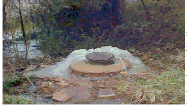
Sanitary sewer overflow into creek
