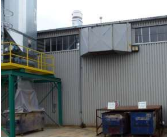
Figure 4: Dust extraction system at NE2 (left) and spare hoppers (right)
