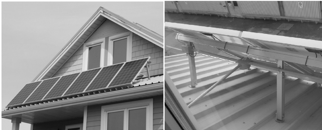
Figure 5: Array Support Frame for Retrofitted PVs
