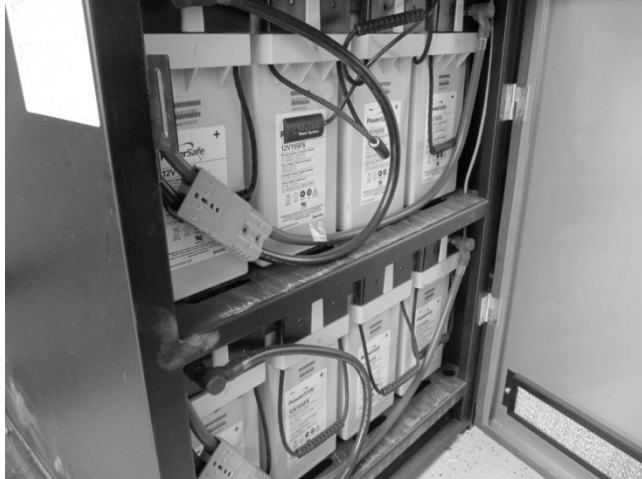
Figure 9: GridPoint Appliance Batteries
