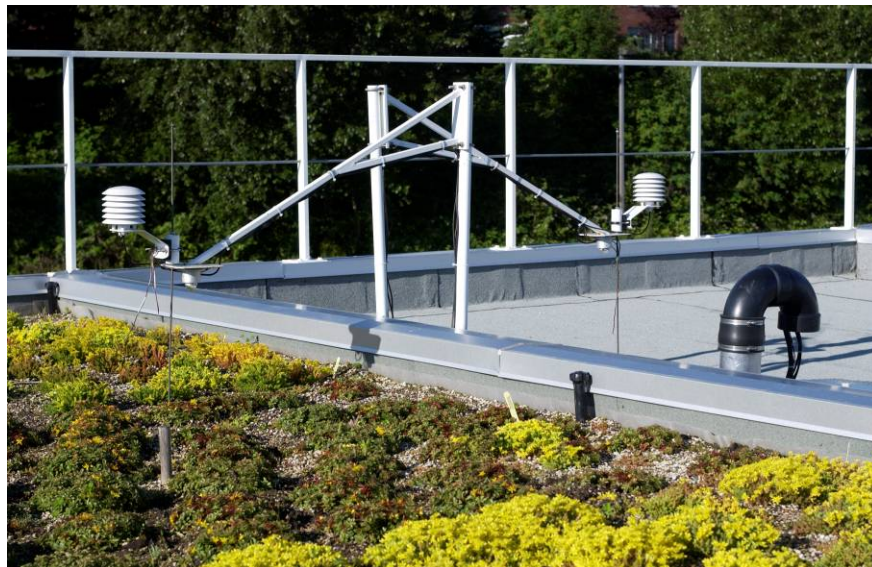
Photo 14 BCIT Green Roof Research Facility weather pole, including solar radiation sensor, relative humidity and temperature transmitter, and thermocouples.
