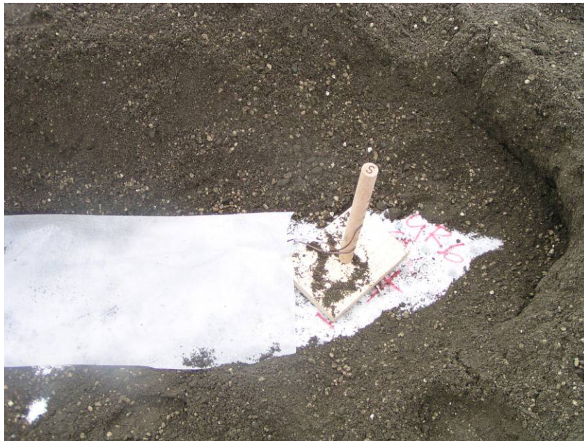
Photo 12 BCIT Green Roof Research Facility instrumentation test point; thermocouples installed in the growing medium.
