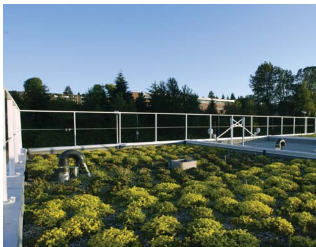
The BCIT Green Roof Research Facility green roof. Photo courtesy of Maureen Connelly
