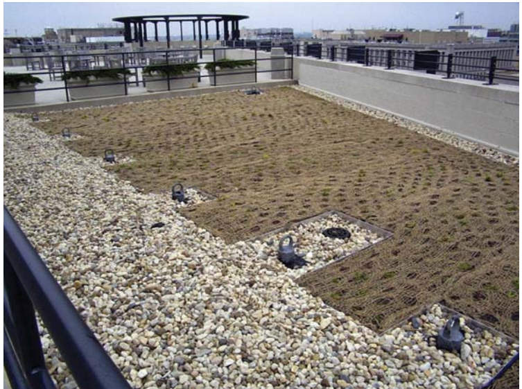
The 1425 K Street green roof, after planting. Photo courtesy of D.C. Greenworks
