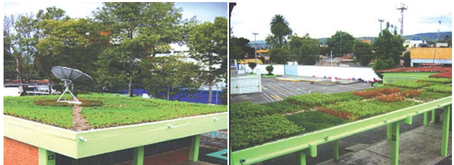
Quilaztli public school after roof greening, Mexico City, Xochimilco Photo: Dr. Gilberto Navas Gomez
