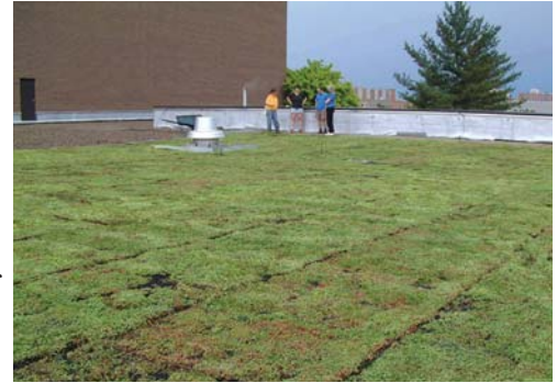
Plant and Soil Sciences Building, Michigan State University. Instrumentation will record data to develop a model for energy consumption.
